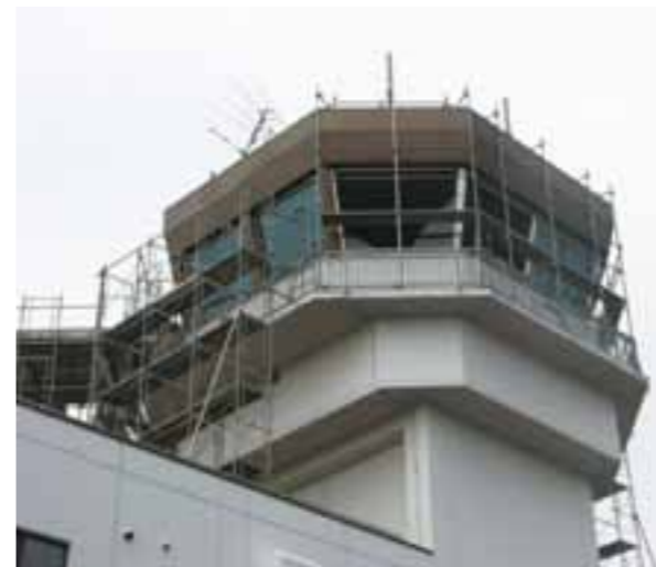
The tower with broken window 导航塔上的窗户已经破烂
